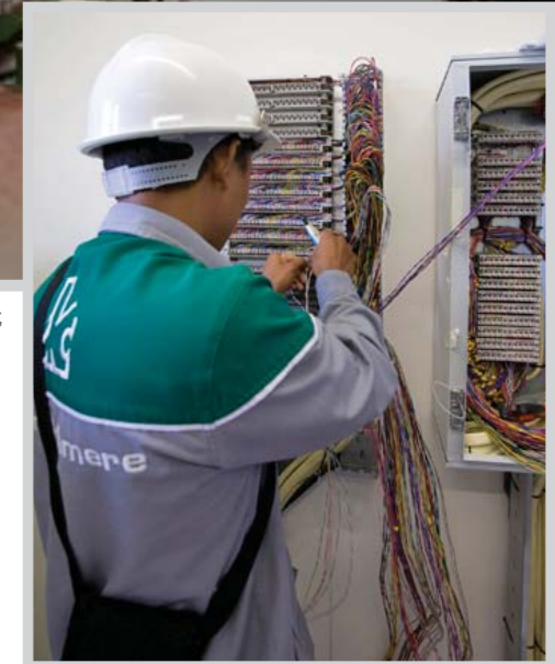
05 | Telephone MDF Panel - Sonja Kill Project
