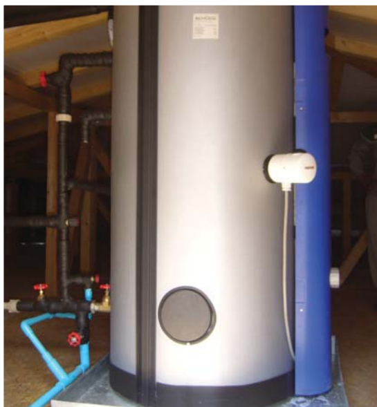
02 | Solar Heating System Storage Tank at German Embassy
