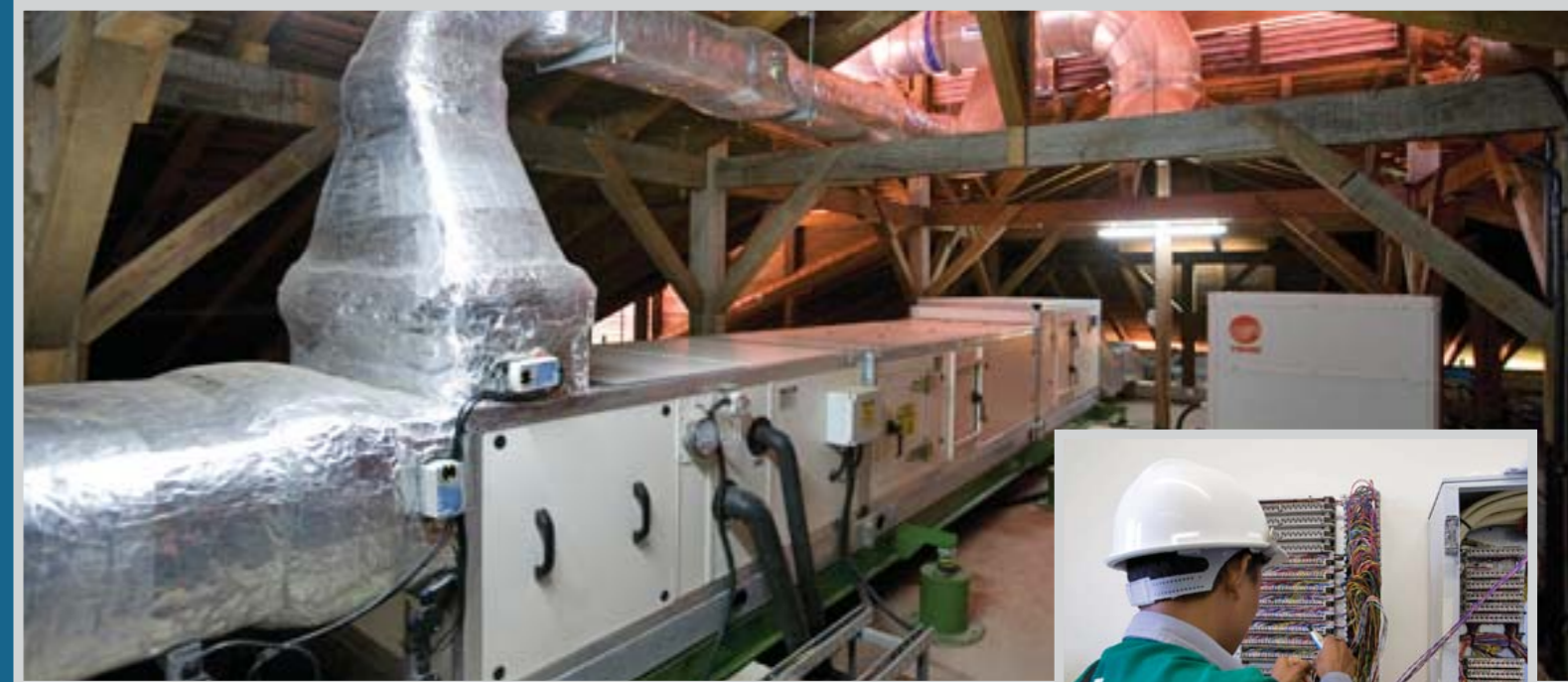
04 | Air Unit for Clean Room- Sonja Kill Project
